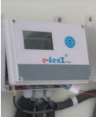
Directly Mounted on wall
