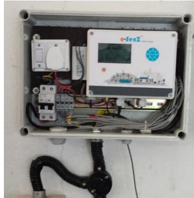
Mounted in Additional IP65 Box
